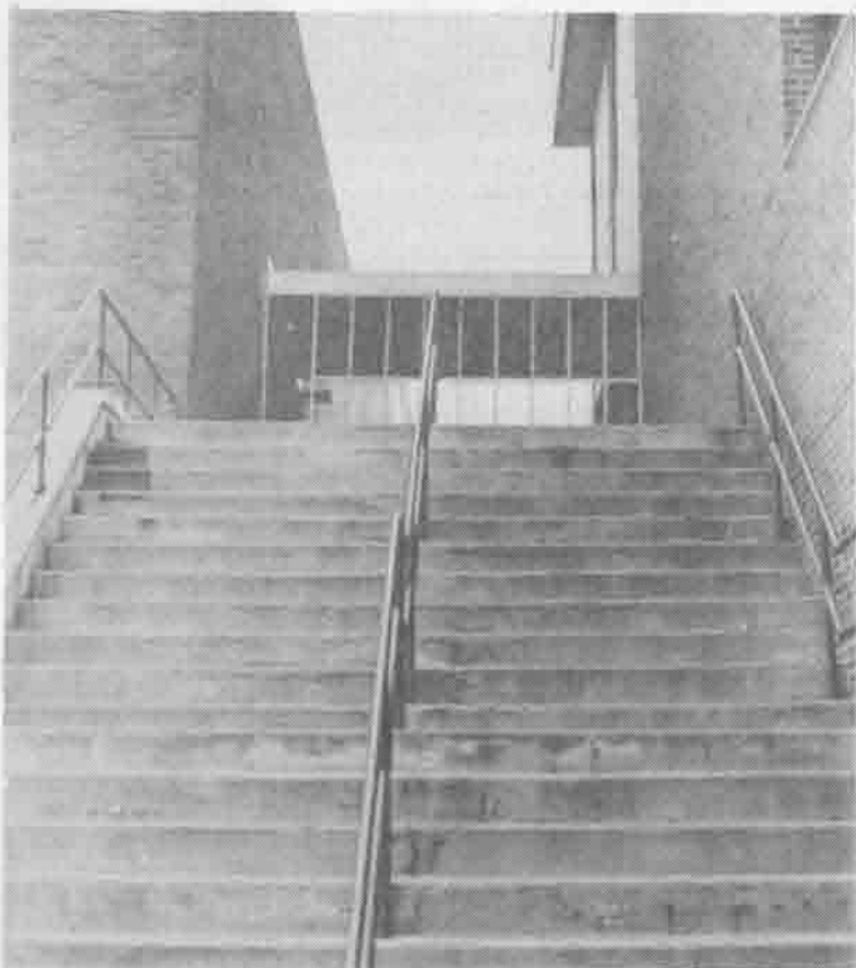
STAIRWAY TO NOWHERE: One of the most used stairways on campus was closed over Winter break. [photo by Earl Swift].
